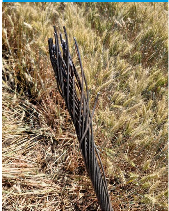
Figure 6.2: Photo of the end of the conductor
