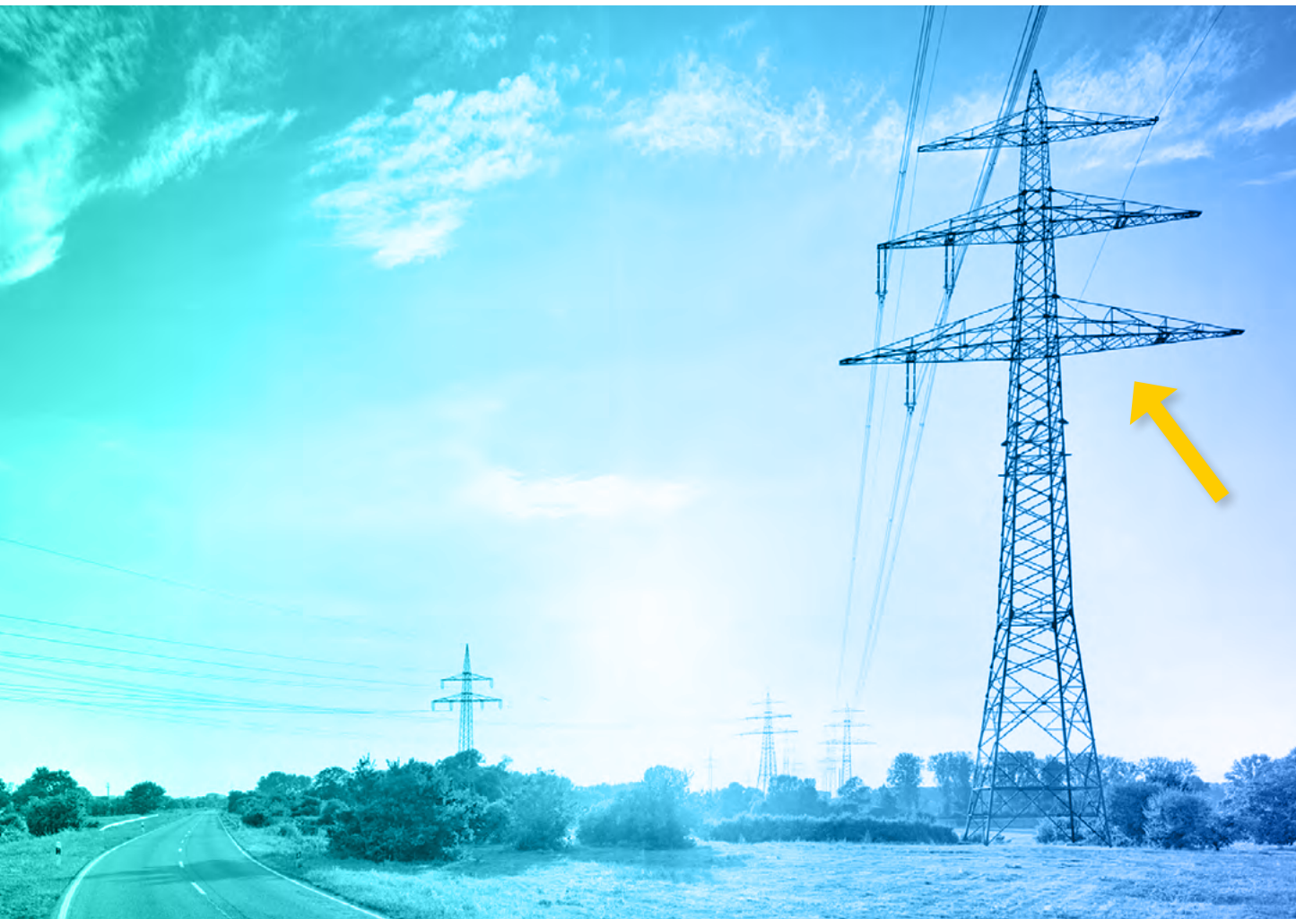
Figure 2: Double-circuit pylons with a single circuit installed as an example for a line which can be easily equipped with an additional circuit
